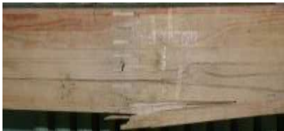
Fig.3. Fracture of the GLB-1
