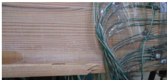
Fig.4. Fracture of the GLB-3
